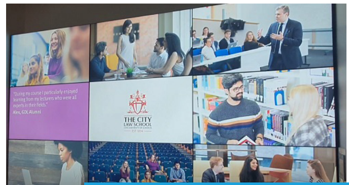
The project required an install of a 3x3 video wall which is displayed in the reception area.
